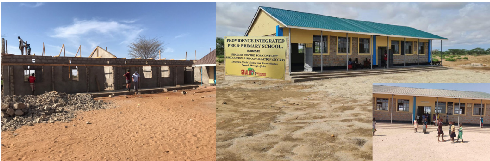
Shalom-SCCRR's Executive Director, Rev. Dr. Oliver Noonan and Mr. Ciaran King, witnessing an ongoing construction of classrooms funded by Shalom-SCCRR in Turkana County, Kenya. On the right, are the completed classrooms.
